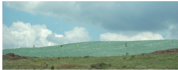
Pictured above is a section of the landfill where geo-membrane liner has been installed.
