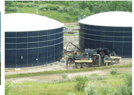
Imperial's leachate tanks collect liquid generated from waste decomposition.
